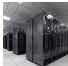
Telecom/IT and Data Centres
